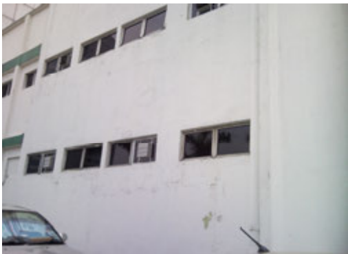
Photo 4 Another view of high humidity or dampness causing mildew/algae/fungi growth near toilet area...
