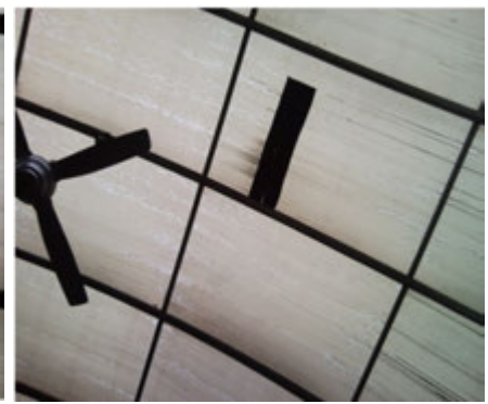
Photo 6 Another view of defective polycarbonate skylight view
