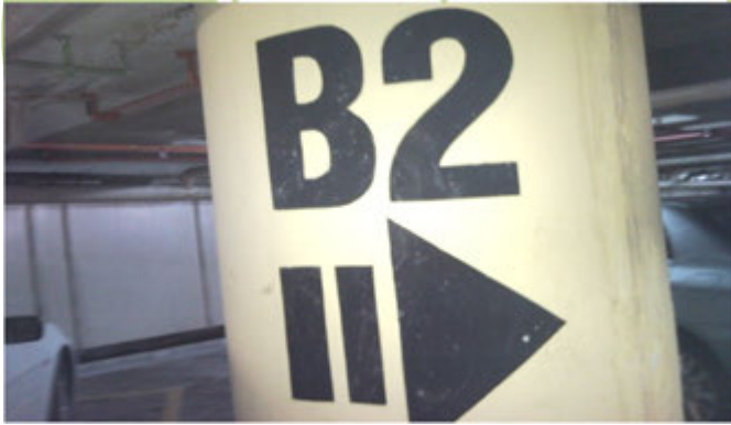
Photo 1 Car park basement B2 m/s c. l. pipes leakage
