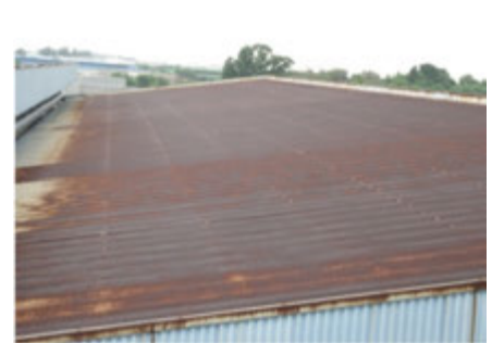
PHOTO 6 Another view of defective metal roof
