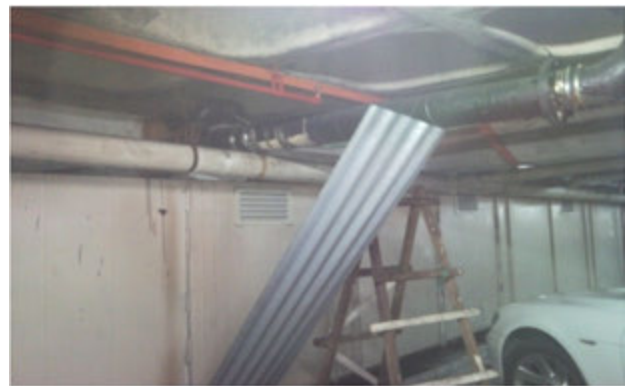
Photo 6 Front view of leakage piping
