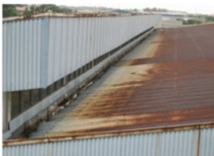
PHOTO 7 Ceiling water stained from metal roof leakage view
