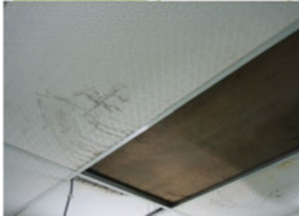
PHOTO 1 Ceiling water stained from metal roof leakage view
