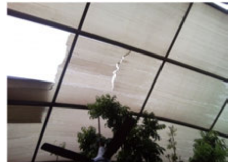
Photo 9 Garden Dome site cracked polycarbonate view
