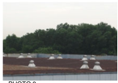
PHOTO 9 Side view defective metal roof
