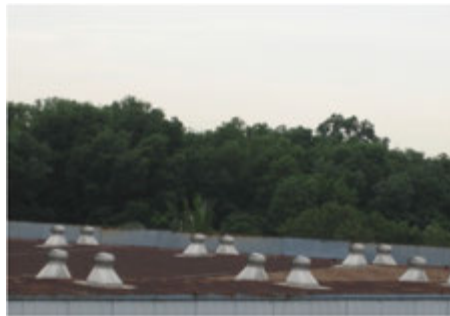
PHOTO 5 Top view of defective metal roofing
