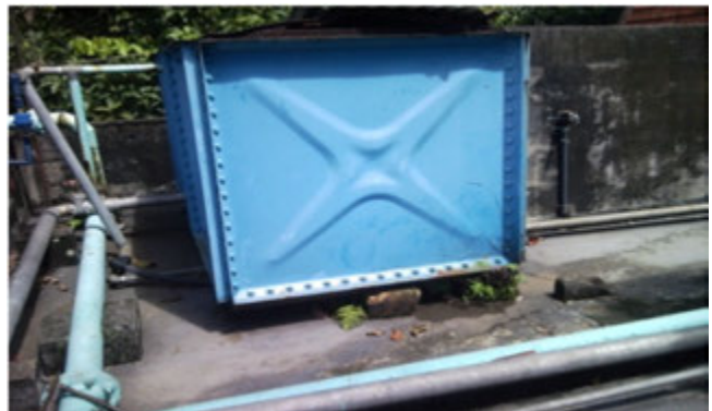
Photo 6 Another view of smaller water tank corroded view
