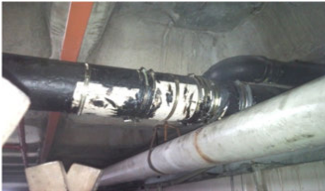
Photo 3 Side view of c.l. piping leakage at car park B2 area
