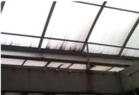
Photo 4 Side view of defective polycarbonate skylight view
