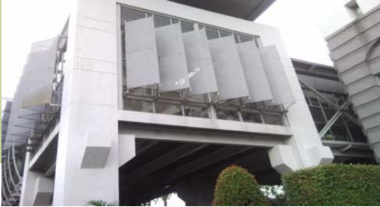
Photo 1 Hotel Glass Window Cleaning System
