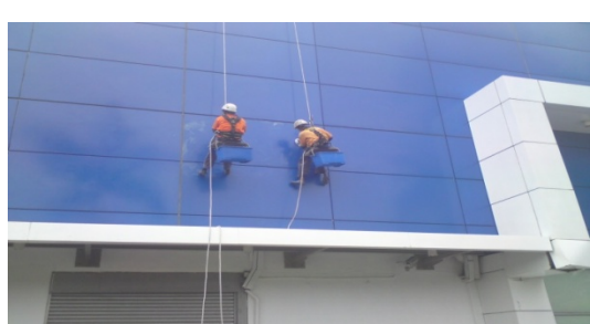
Photo 8 Hypermarket exterior window and panel cleaning system
