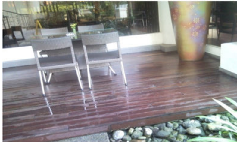
Photo 4 Another view of defective flooring deck
