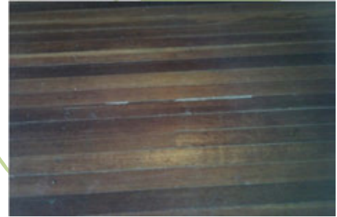
Photo 3 Banquet Hall wooden flooring defective view
