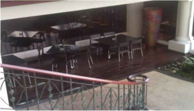
Photo 1 Front View of Kites Restaurant exterior defective floor deck
