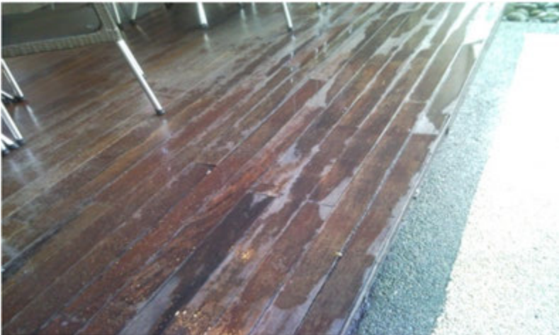
Photo 3 Kites Restaurant defective flooring deck view
