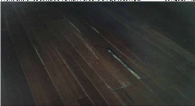
Photo 4 Another view of defective flooring at Banquet Hall
