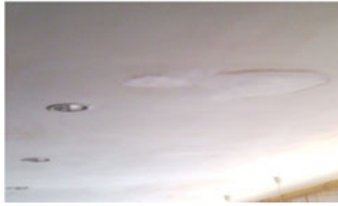
Photo 5 interior ceiling stained due to leakage from above metal roof..
