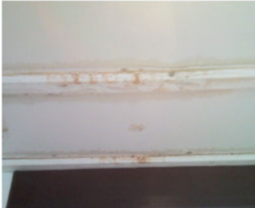
PHOTO 5 Room entrance door frame ceiling board water stained view
