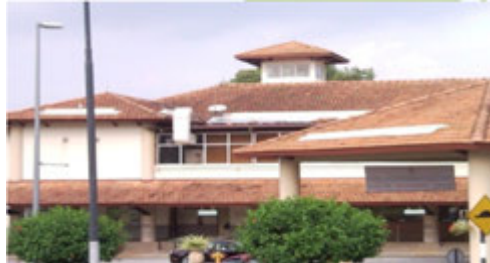
Photo 2 Existing external tile and metal roof leakage view
