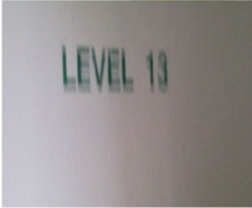
PHOTO 2 Level 13 tower block to room RC slab leakage
