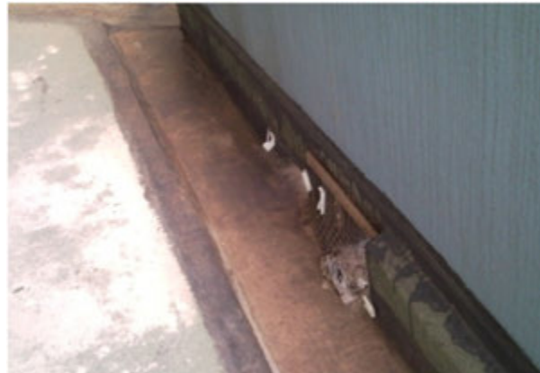
c. Defective scupper drain, causing leakage to below Spine & Joint Center.
