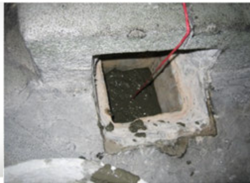
i. Thereafter to fill Cement top up about 1 inch to seal the opening in progress...
