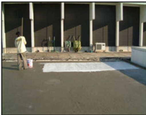
4. Application of cementitious membrane to strengthen existing surface followed by 3 coat of liquid applied membrane.
