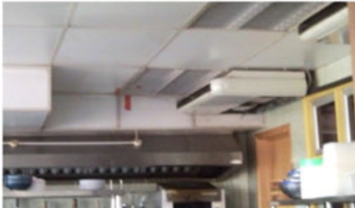
Photo 4 Japanese restaurant kitchen area leakage from above metal roof
