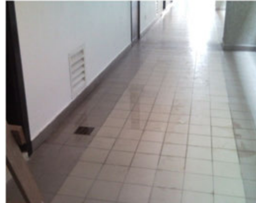
PHOTO 6 Room entrance floor water stained due to leakage from above RC slab
