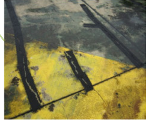
PHOTO 3 Cracked and defective R.C. flat roof view.
