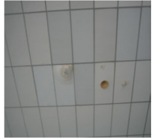
PHOTO 6 Water stained mark at ceiling board from roof top view.
