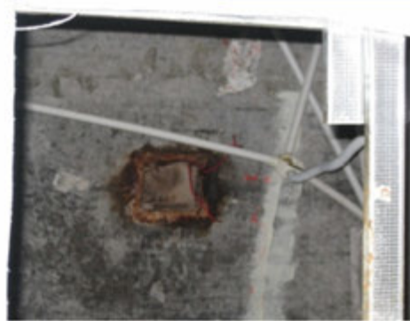
b. Leakage spot can be seen at opening soffit area.
