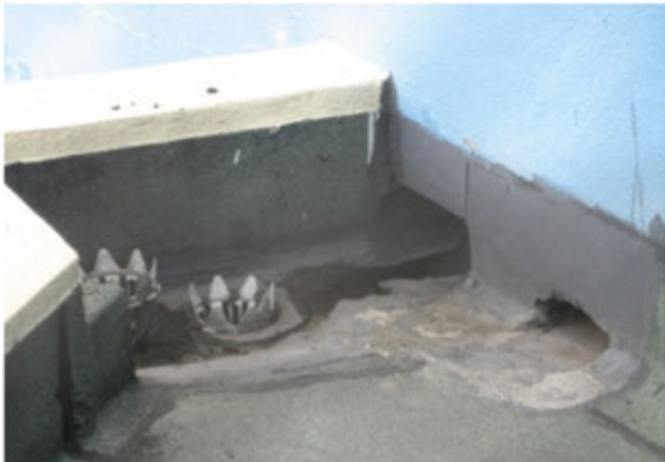
d. Another view of scupper drain defective causing below Spine & Joint Centre water seepage problem
