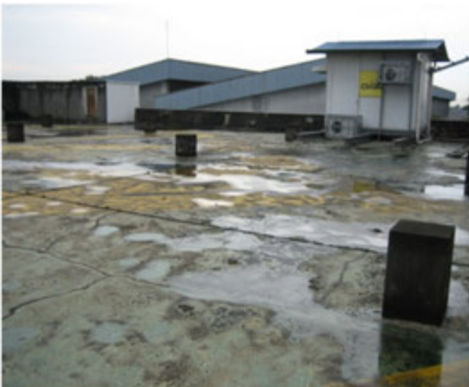
PHOTO 4 Water ponding and defective R.C. flat roof view.
