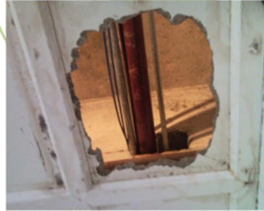
PHOTO 3 Level 13 room entrance above RC slab leakage to below ceiling board view
