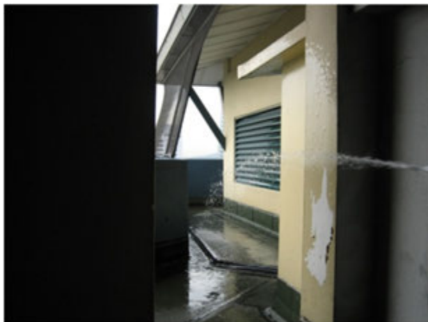
f. After completion the treated area, thereafter to conduct water testing at site. Result OK.
