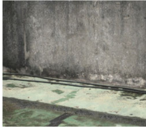
PHOTO 5 Another view of defective R.C. flat roof and parapet.
