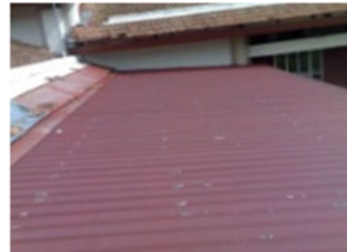
Photo 9 Metal roof top view of defective flashing between tile roof and metal roof joint..
