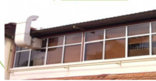
Photo 3 Another view of metal roof front elevation where leakage from metal roof top
