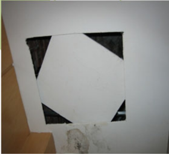
a. 7th Floor Spine & Joint Centre another water seepage stained problem at location 2
