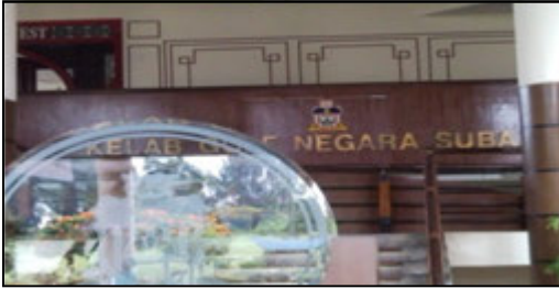
Photo 1 Kelab Golf Negara Subang entrance to Japanese Restaurant roof leakage..
