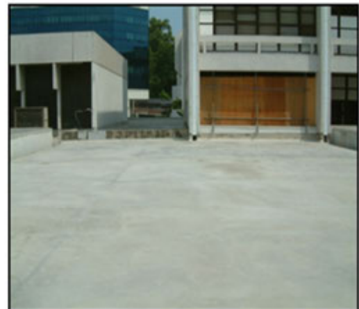
8. Completion of build up waterproofing system to old RC Roof. Completed in September 2003.
