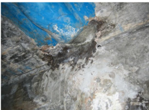
e. Application of high strength epoxy putty to seal the leaking spot.
