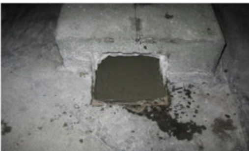
l. Another view of non-shrink grout to render level at roof top area.
