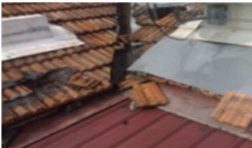
Photo 11 Flashing not cover to the extended valley and joint area between tile and metal roof and defective sealant to be treated to avoid water backflow
