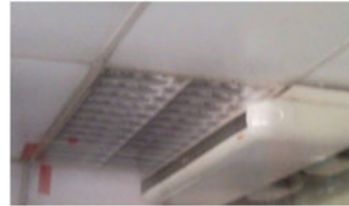
Photo 6 Another view of ceiling stained
