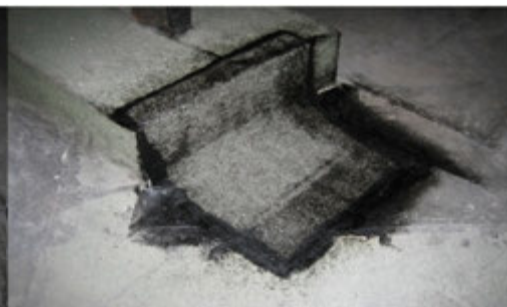
m. After curing, to replace a new membrane at the localise repair and make good.
