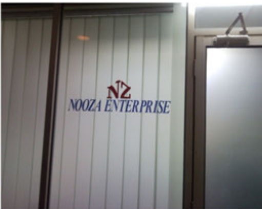
PHOTO 7 Another location at NOOZA ENTERPRISE office water stained view
