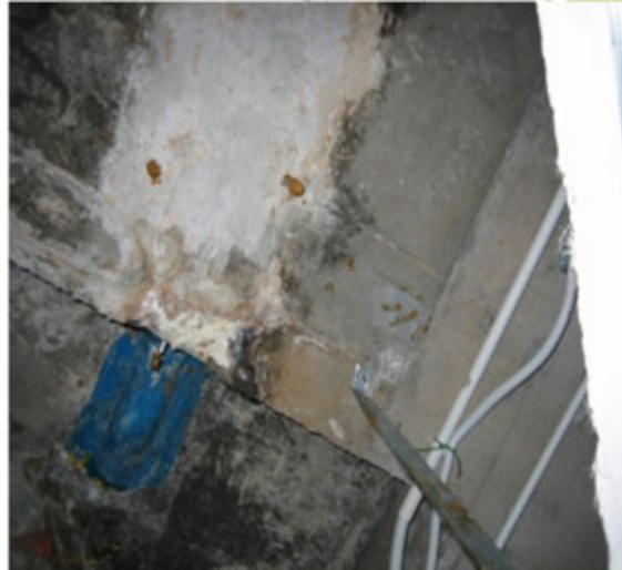
b. leaking location view at location 2
