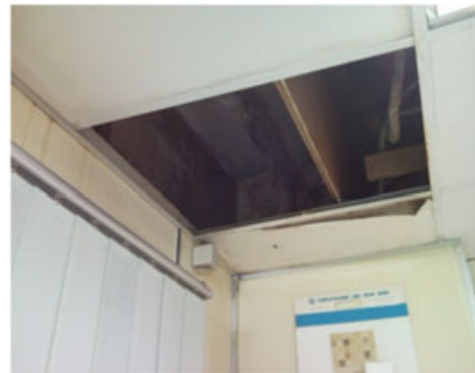
PHOTO 9 Another view of NZ RC slab stained view
