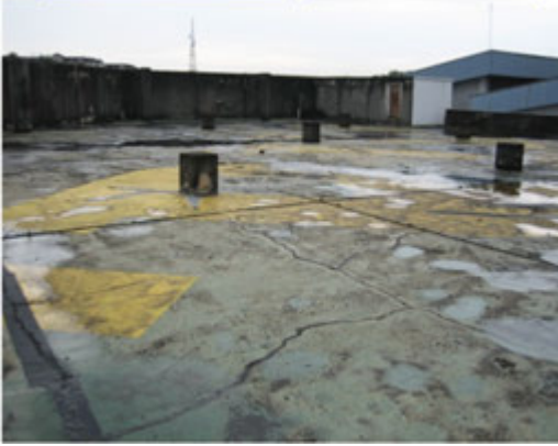
PHOTO 1 Top view of defective R.C. flat roof at block A office area
