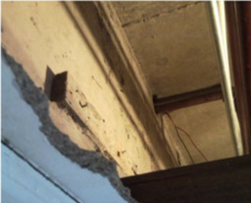
PHOTO 4 Level 13 room entrance RC slab leakage and causing below stained
