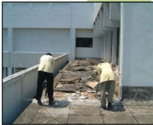
2. Hacking of existing panel, insulation board, separation layer and existing waterproofing membrane.
