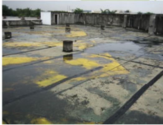
PHOTO 2 R.C. flat roof water ponding view
