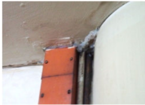
Photo 7 Kitchen area stained ceiling and wall area due to leakage from above metal roof
