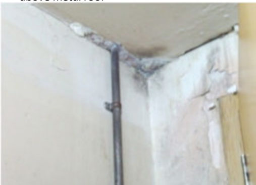
Photo 8 Interior kitchen area water stained from above metal roof. Flashing not cover to the extended valley and joint area between
