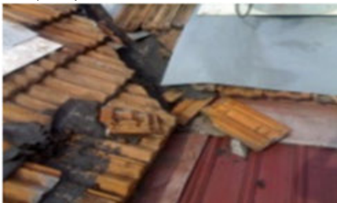
Photo 10 Top view of defective tile and valley area causing heavy rain water back flow to ceiling area....
