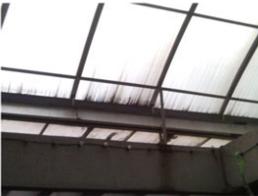
Photo 4 Side view of defective polycarbonate skylight view
