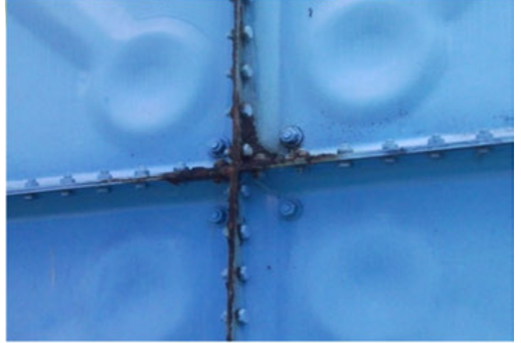
Photo 2 Corroded exterior water tank view
