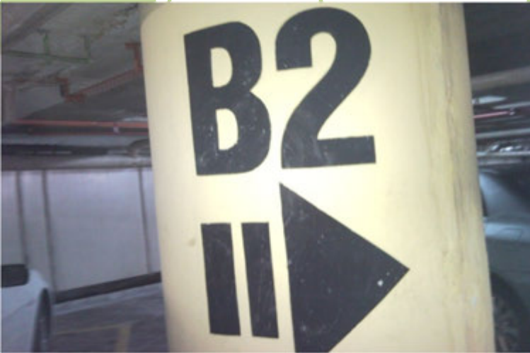
Photo 1 Car park basement B2 m/s c. l. pipes leakage
