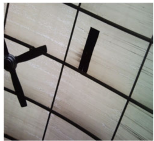
Photo 6 Another view of defective polycarbonate skylight view
