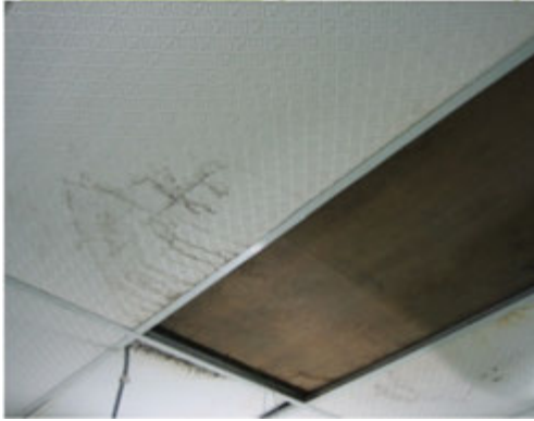
PHOTO 1 Ceiling water stained from metal roof leakage view
