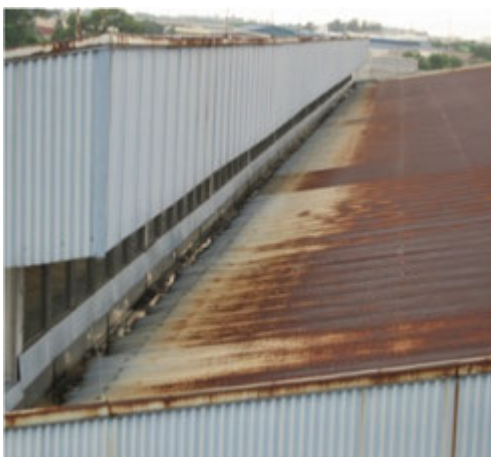
PHOTO 7 Ceiling water stained from metal roof leakage view
