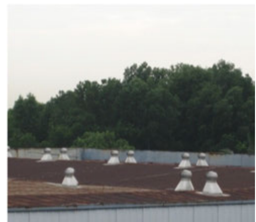
PHOTO 9 Side view defective metal roof
