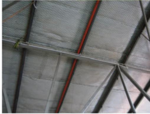
PHOTO 2 Water stained From above metal roof defective view
