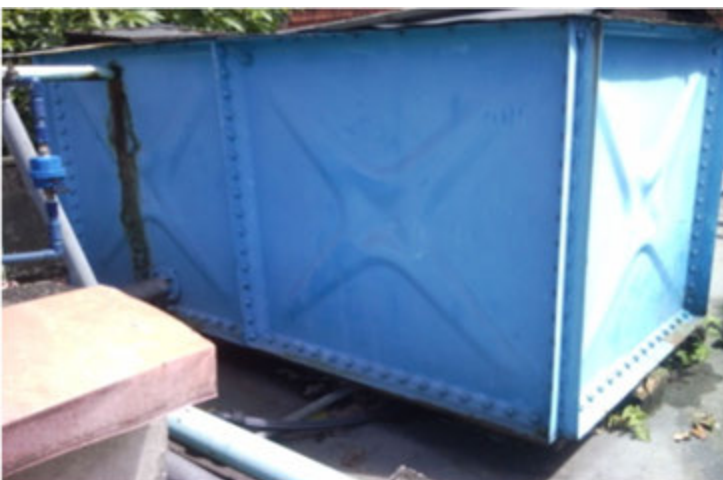
Photo 5 Smaller water tank view
