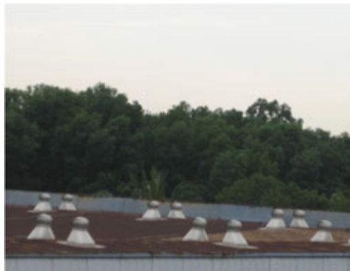
PHOTO 5 Top view of defective metal roofing
