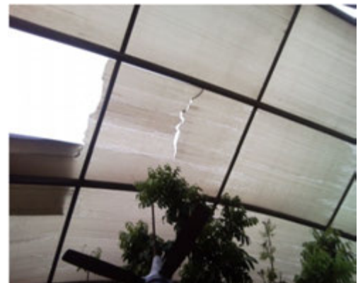
Photo 9 Garden Dome site cracked polycarbonate view
