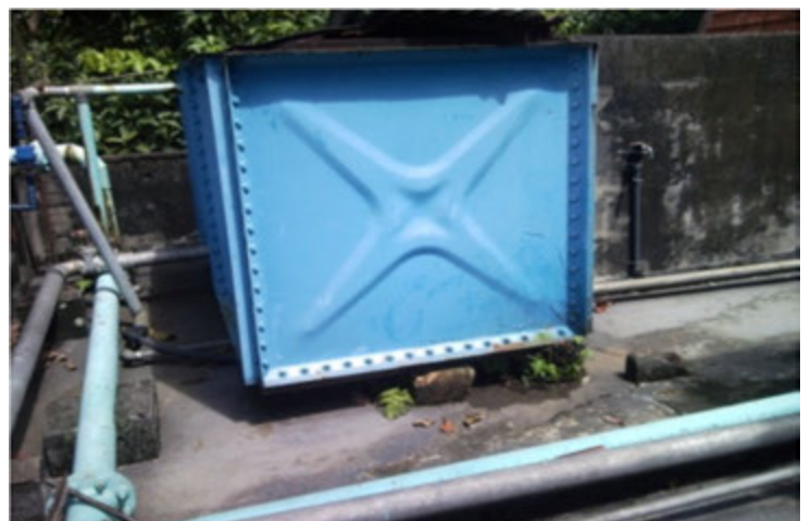
Photo 6 Another view of smaller water tank corroded view
