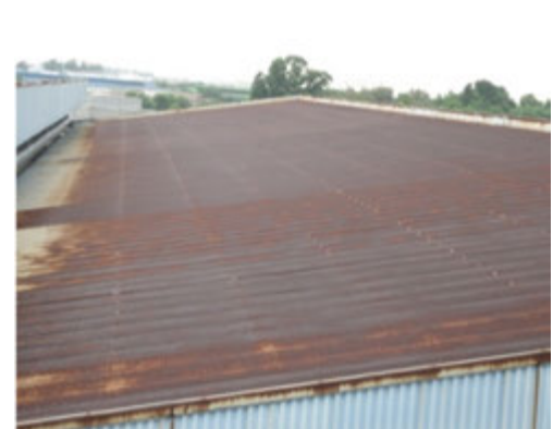
PHOTO 6 Another view of defective metal roof
