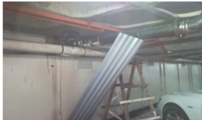
Photo 6 Front view of leakage piping
